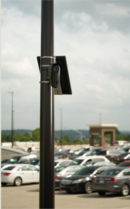
Solar & Existing Pole
